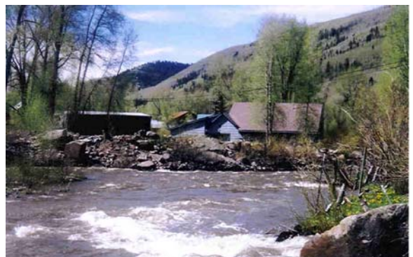
Figure 2-8: Broken concrete, rubble and dirt have been bermed up to protect these houses from flood hazards. Berms adjacent to the river destroy riparian vegetation and concentrate stream power on the channel during a flood thereby reducing stability.
