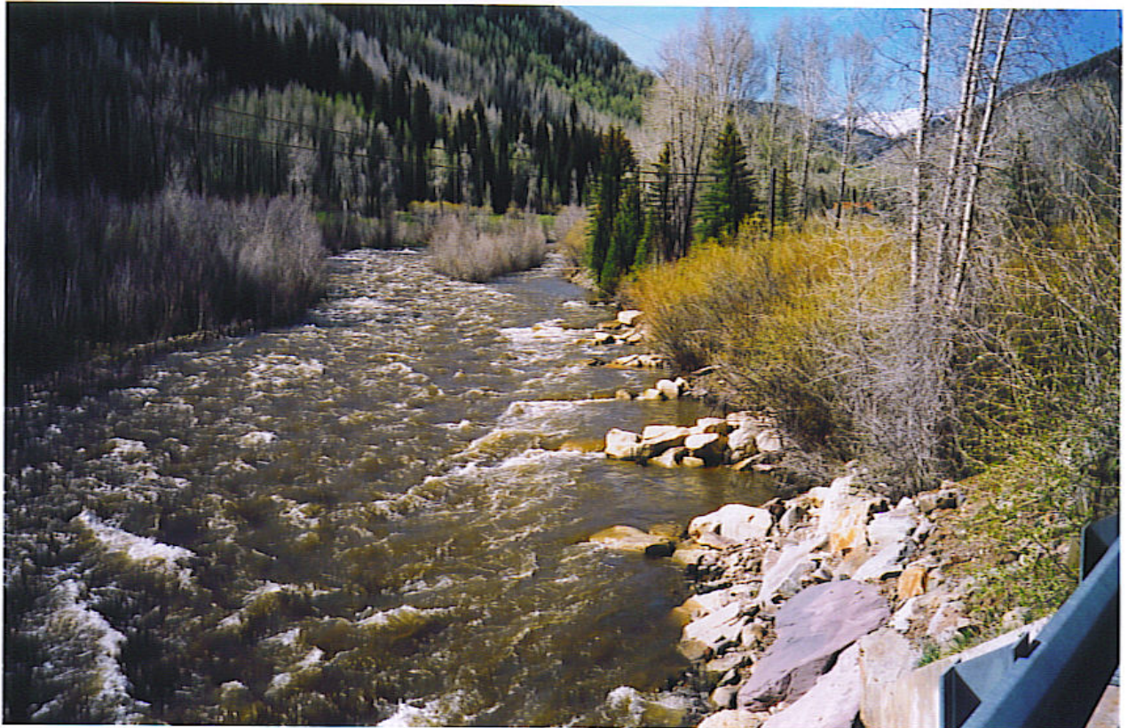
These seven diverter spurs angled downstream were constructed along the east bank of the Dolores River near the town bridge to keep the river back in the existing main channel location and prevent it from creating a flow path around the bridge.
